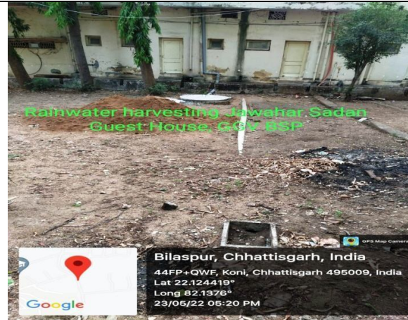
Rain Water Harvesting @ Jawahar Guest House
