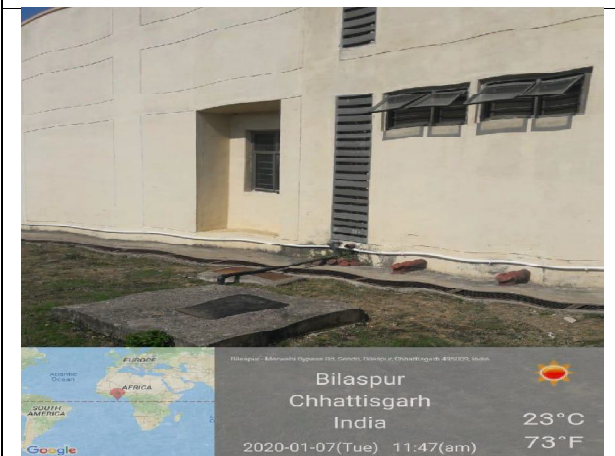
Rain Water Harvesting @ New Boys Hostel – A (Back Side)
