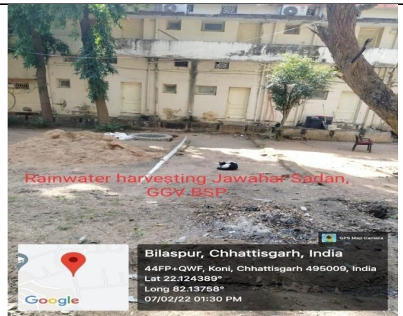
Rain Water Harvesting @ Jawahar Guest House
