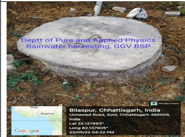
Rain Water Harvesting @ Physics Department
