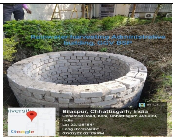
Rain Water Harvesting @ Administrative Building
