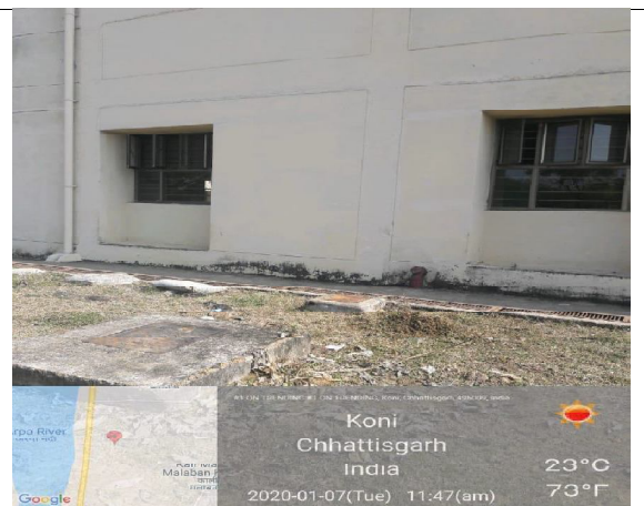
Rain Water Harvesting @ New Boys Hostel – B
