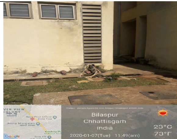
Rain Water Harvesting @ New Boys Hostel – A
