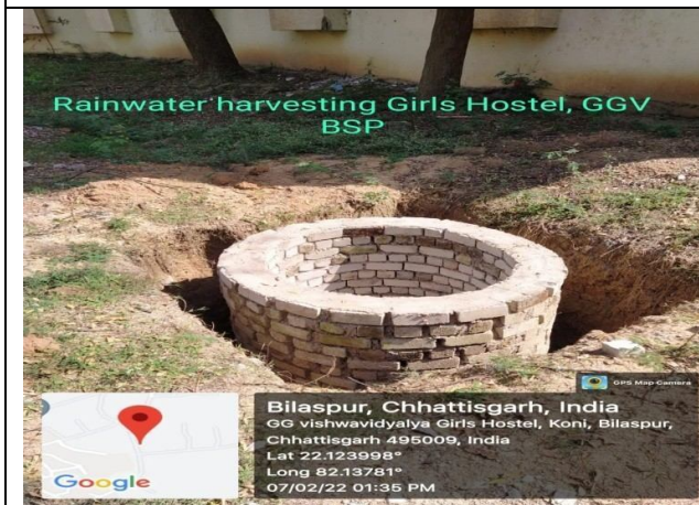
Rain Water Harvesting Girls Hostel
